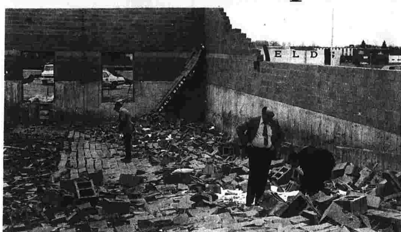
Men inspect the debris inside the sixth Showcase Cinema theater in East Hartford only minutes after wind toppled the wall at the right onto two men preparing the concrete floor this morning. (Herald photo by Pinto)
